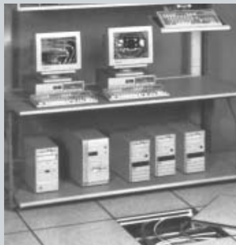
COMPUTER ROOMS/DATA CENTERS
